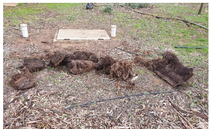
Figure 2 roots clogging up septic tank
